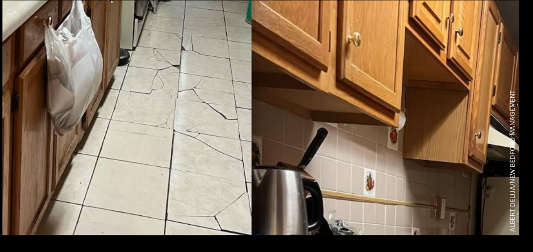
Warning signs: Cracked tiles and tipping wall cabinets revealed major structural issues at the Crown Heights co-op.
